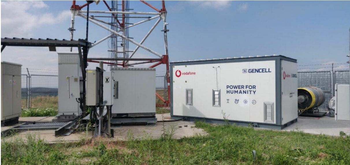
Figure 8: A GenCell FOX™ ammonia-based off-grid power solution in Romania
